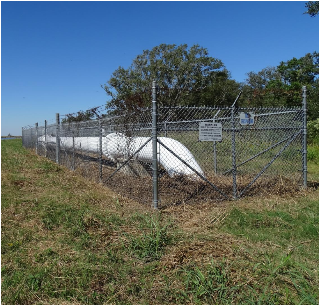
West Pumping Facility
