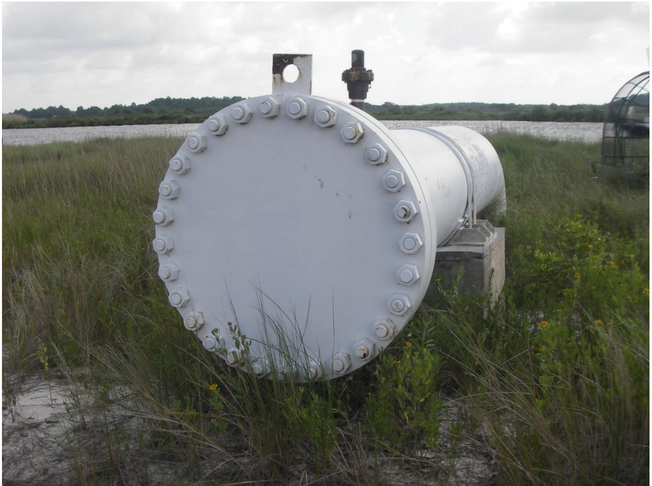
West End Blind Flange/Riser Pipe
