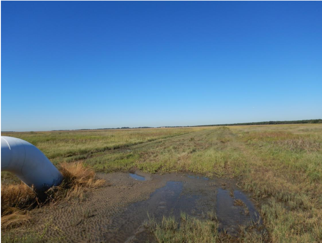
Pipeline Corridor (View from East Blind Flange looking West Towards LA HWY 27)
